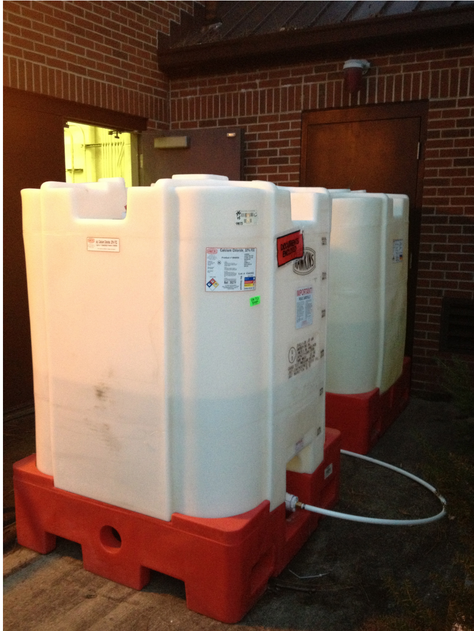
Figure 18: Brine solution tank.
