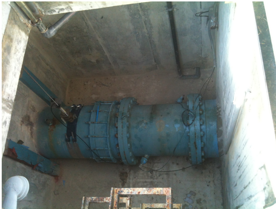
Figure 17: Flow meter and injection pipe main outlet.
