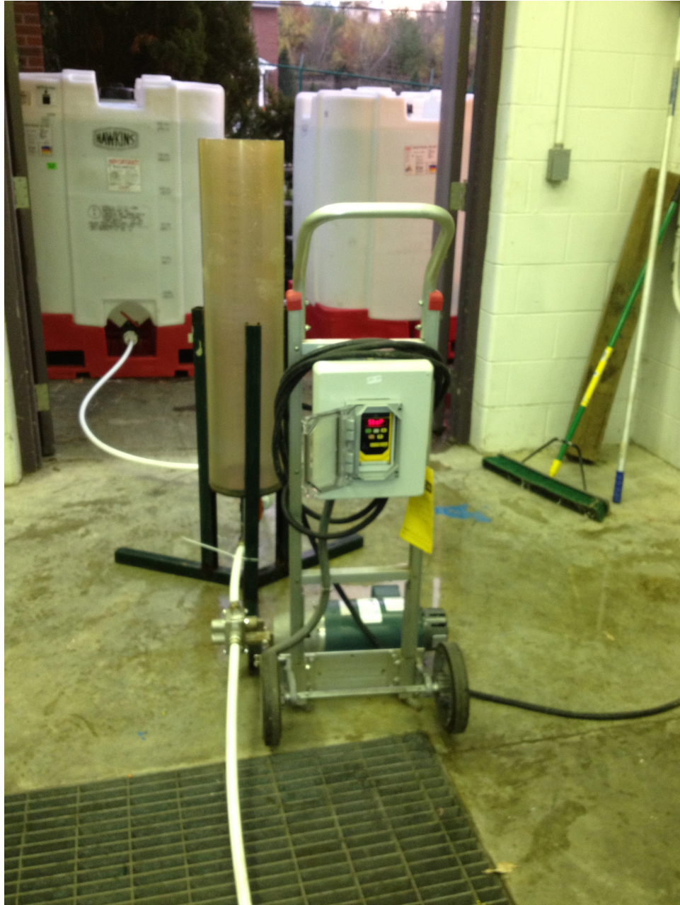
Figure 19: Brine injection pump with volumetric flow measurement device.
