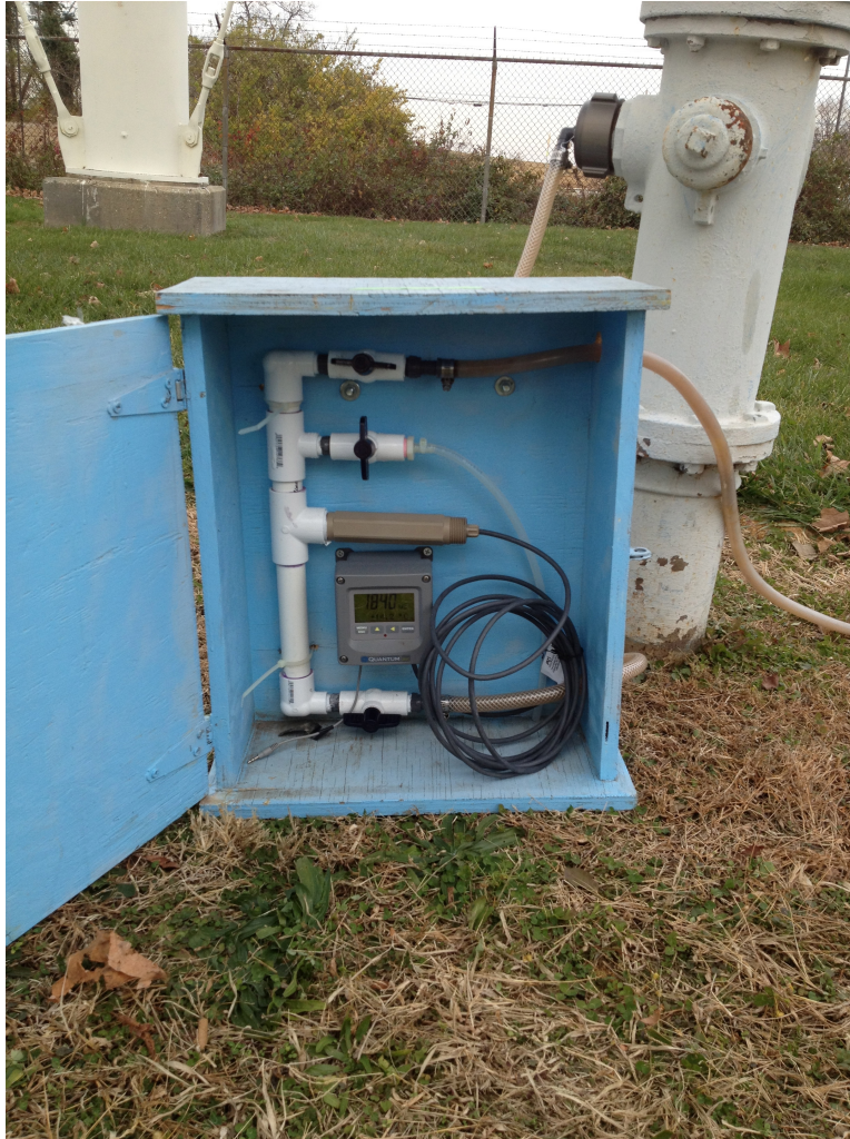
Figure 9: Continuous conductivity and temperature analyzer and grab sample tap (typical).
