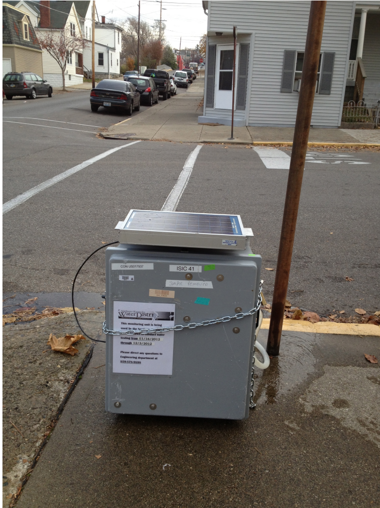
Figure 7: Continuous conductivity and temperature analyzer and grab sample tap (typical).
